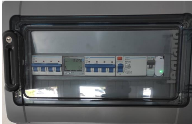
Figure 21: Indicative challenges in electrical boards of households in the Greek pilot
